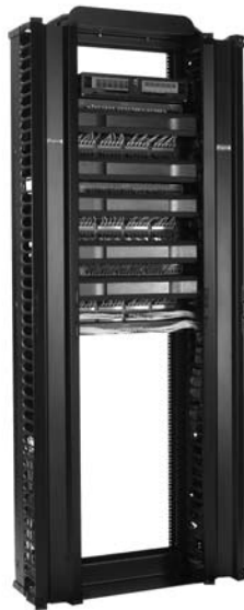
Populated Two-Post Rack with vertical cable management
